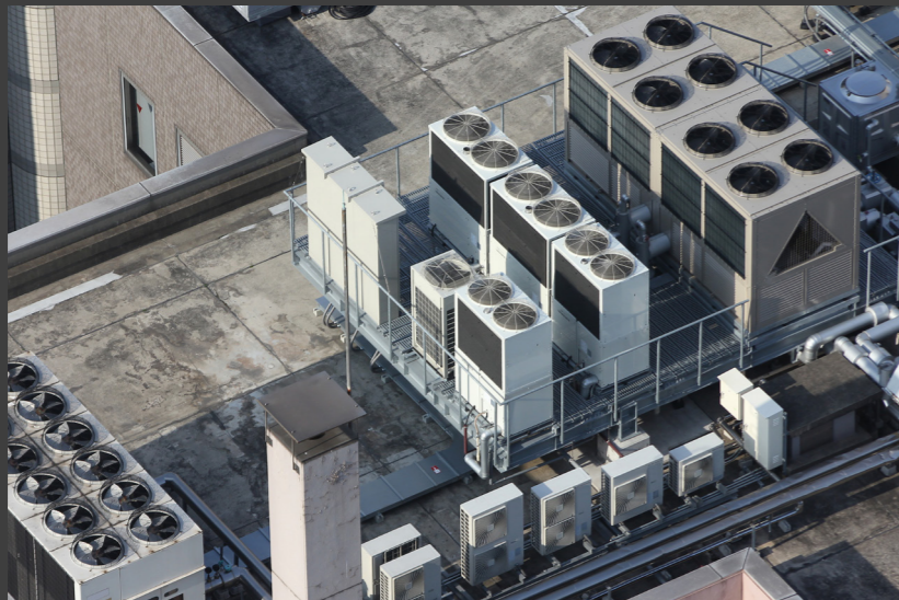
Motor and temperature control
